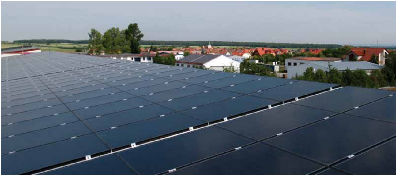
This rooftop installation on the BELECTRIC warehouse is a successful example of how to use industrial rooftops for ecological power generation. (Image: BELECTRIC)
